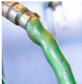
Old coupling with hose clamps causing leakage and pressure drop
